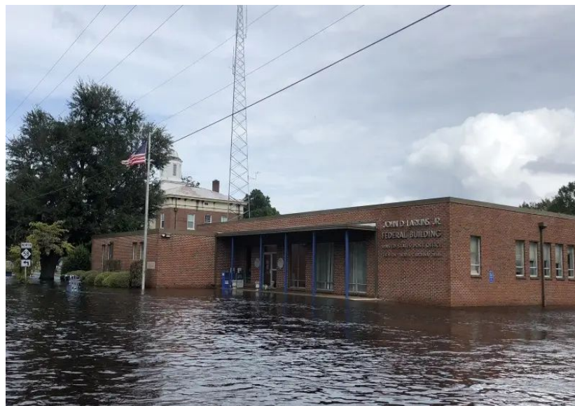
After flooding (photograph)
