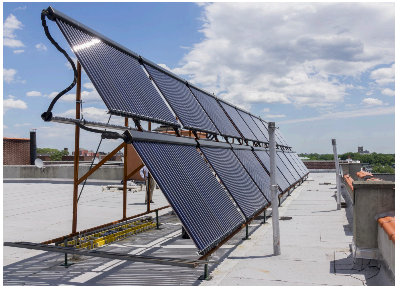
Fordham Bedford Housing Corporation, located in the Jerome Park neighborhood in the Bronx, takes advantage of the Green Housing Preservation Program to make cost-saving green upgrades including a solar infrastructure installation. Source: Housing Preservation and Development
