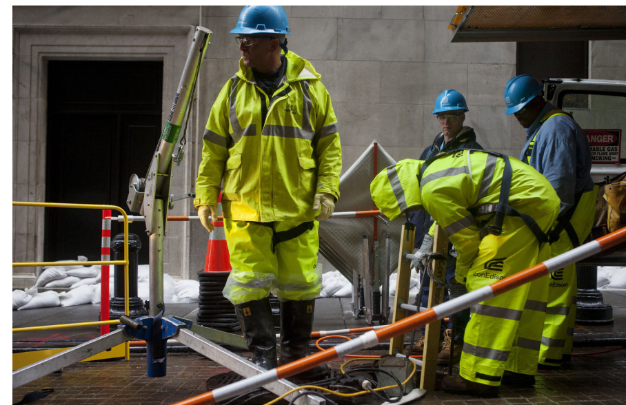
Growing New York City's electric grid is key to supporting the transition from fossil fuels to clean energy. Source: Mayor's Office of Climate & Environmental Justice
