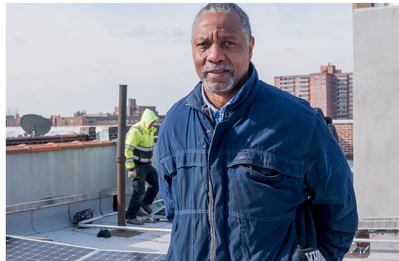
Oral, the landlord of an apartment building in the Flatbush neighborhood of Brooklyn that he inherited from his dad, takes advantage of the Green Housing Preservation Program to make cost-saving green upgrades including a solar infrastructure installation. Source: Housing Preservation & Development
