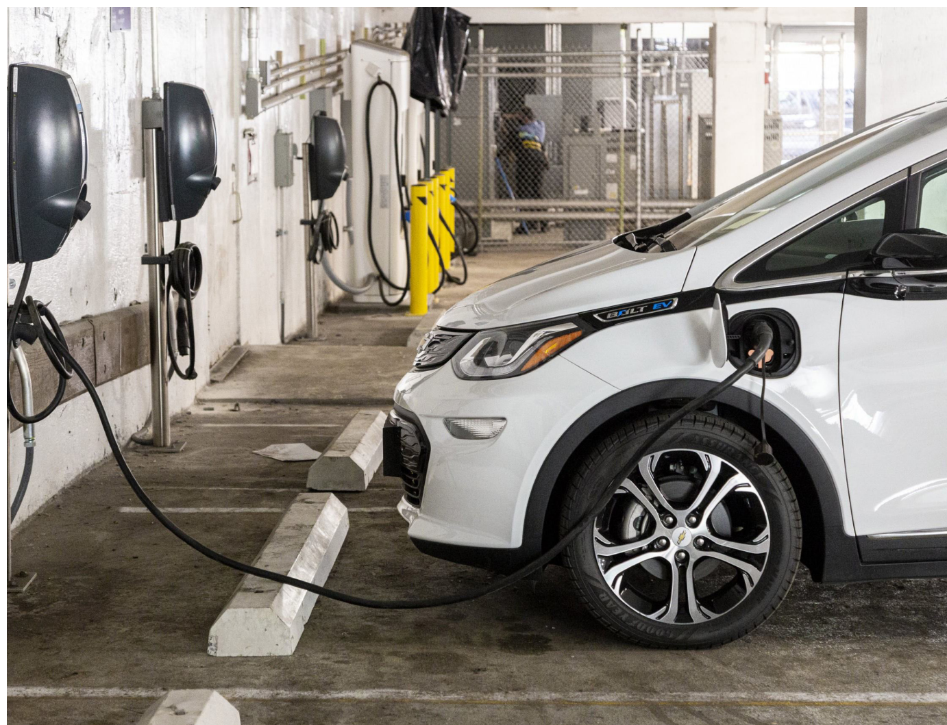
The Department of Transportation's Delancey and Essex Municipal Parking Garage in the Lower East Side neighborhood of Manhattan offers shared electric charging depots, promoting EV use. Source: Department of Transportation
