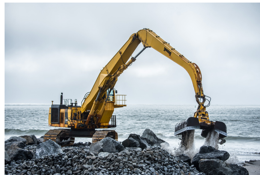
In October of 2022, Mayor Adams broke ground on the Brooklyn Bridge-Montgomery Coastal Resiliency project, which will protect the Two Bridges neighborhood of Manhattan from coastal storm surge through a combination of flood walls and deployable flip-up barriers (top). The U.S. Army Corps of Engineers (USACE) commenced construction on the Atlantic Shorefront Resiliency Project in the Rockaways, Queens (bottom). Source: Mayor's Office
